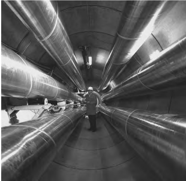
FIGURE 18.15 Tunnel arrangement of two systems GIL for the long-term test. (Courtesy of Siemens AG, Erlangen, Germany.)
