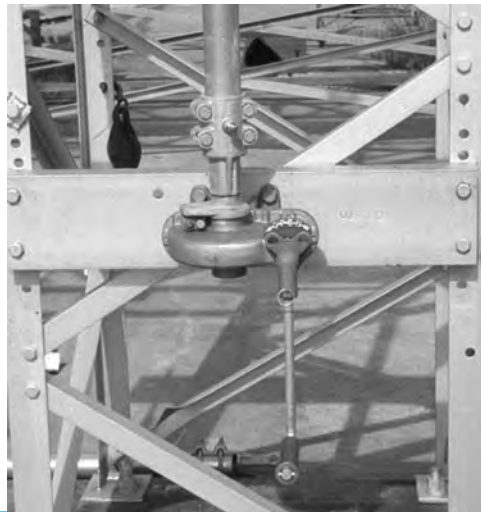
FIGURE 4.5 Gear crank operator for disconnect switch.
