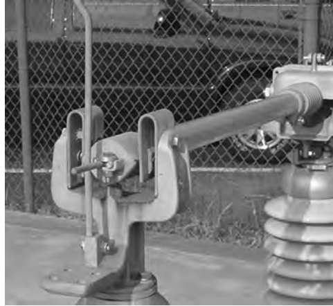
FIGURE 4.25 Arcing horns on a vertical break switch.
