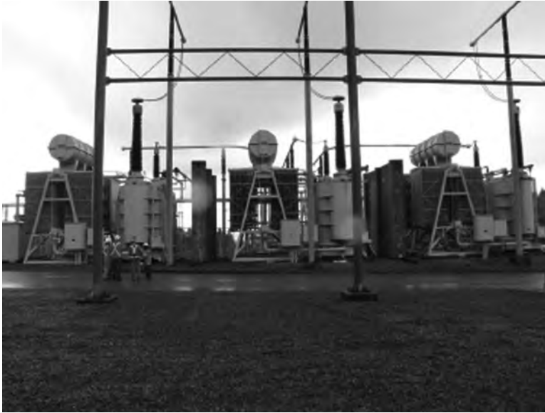
FIGURE 14.4 Fire barriers between individual single-phase transformers that are not high enough to protect the 230 kV bushings on adjacent transformers.
