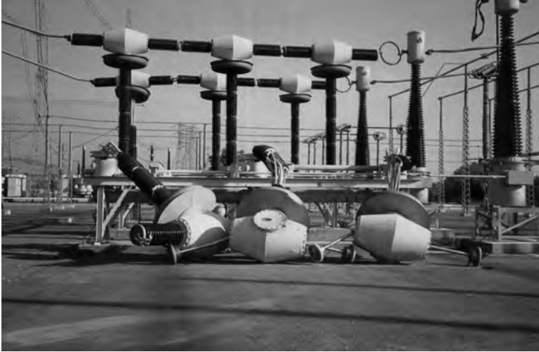
FIGURE 13.1 500kV live tank circuit breaker. (Photo courtesy of E. Matsuda, Copyright 1989–2011 Pacific Gas and Electric Company, Oakland, CA. All rights reserved.)
