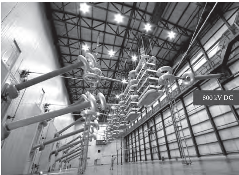
FIGURE 5.12 800kV UHV DC Yunnan–Guangdong—view of the bipolar valve halls with two 400kV systems in series to build 800kV.
