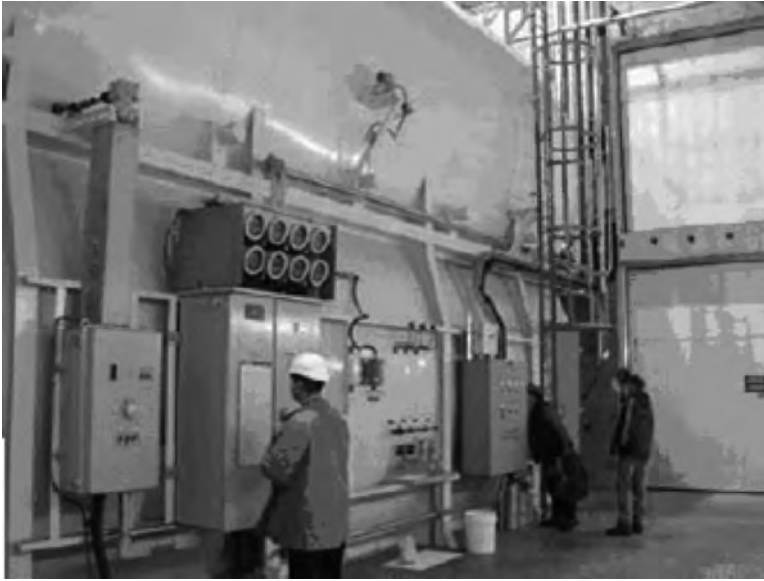
FIGURE 14.1 Shows large distribution transformer in an explosion containment tank inerted with nitrogen.
