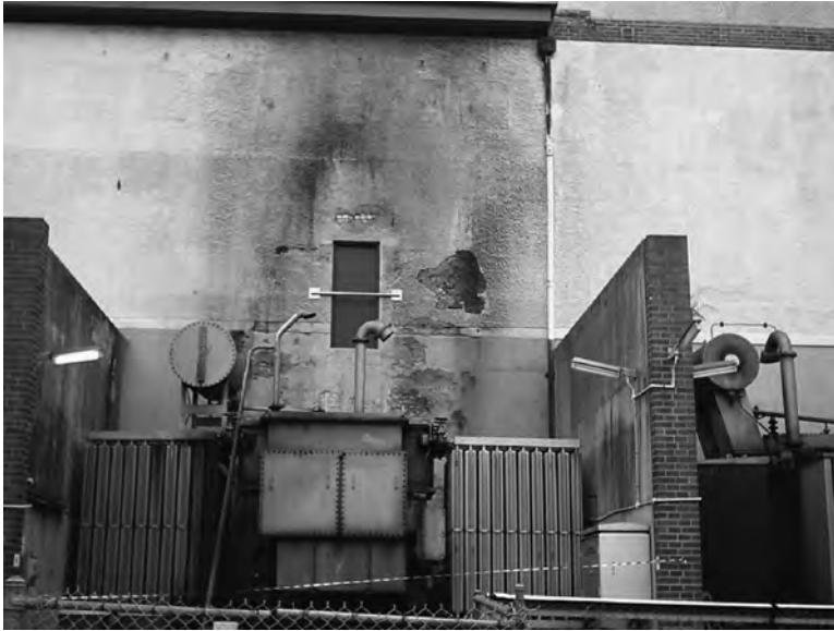
FIGURE 14.2 Shows damage to the wall of substation control building from a transformer fire. The flame reached above the roof and caused the roof structure to collapse into the control room.
