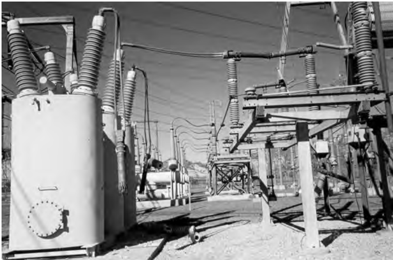
FIGURE 13.4 230 kV circuit breaker and air disconnect switch. (Photo courtesy of E. Matsuda, Copyright 1996–2011 Pacific Gas and Electric Company, Oakland, CA. All rights reserved.)
