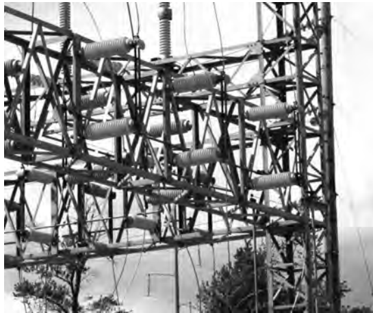
FIGURE 4.9 Vertically mounted disconnect switch.
