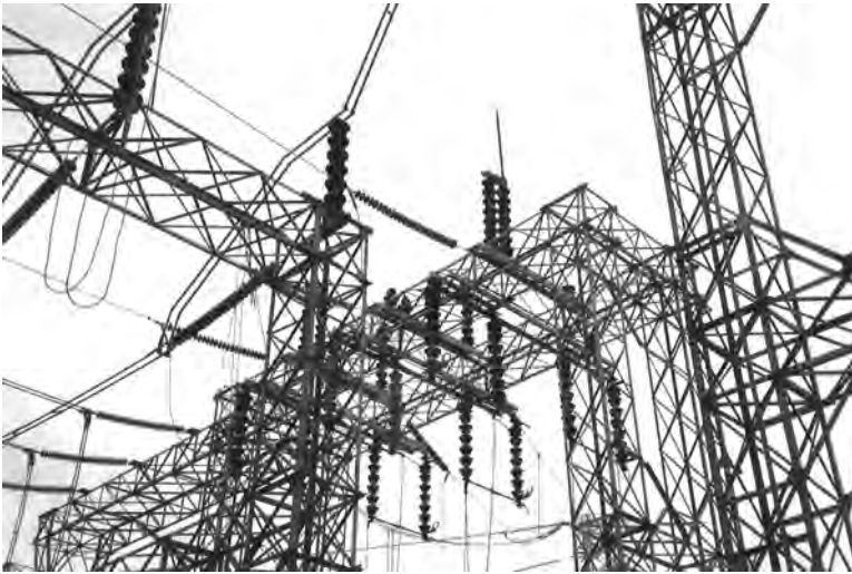
FIGURE 13.2 230kV air disconnect switch. (Photo courtesy of E. Matsuda, Copyright 1989–2011 Pacific Gas and Electric Company, Oakland, CA. All rights reserved.)
