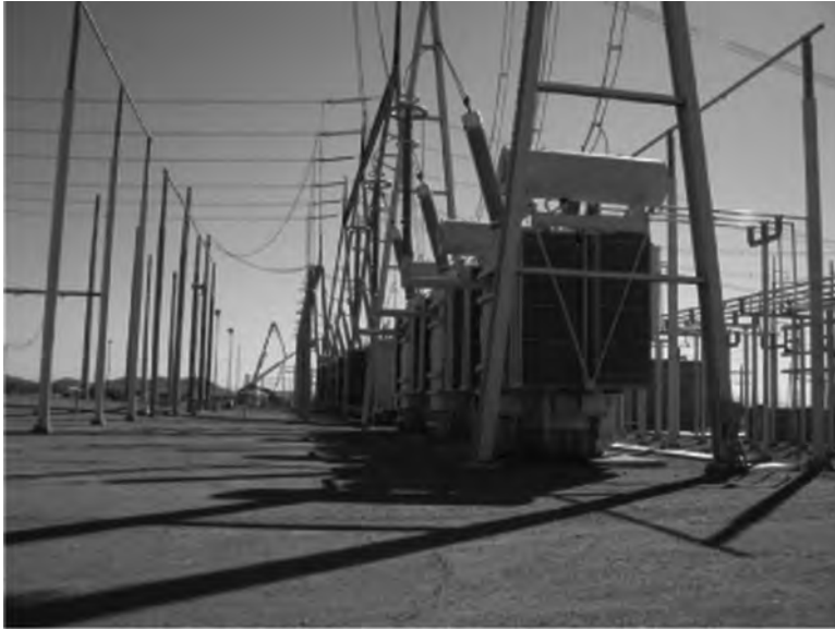
FIGURE 14.3 Shows closely spaced transformer without any fire spill containment or flame suppressing stone. A transformer fire at this substation damaged three additional transformers before the fire was suppressed.
