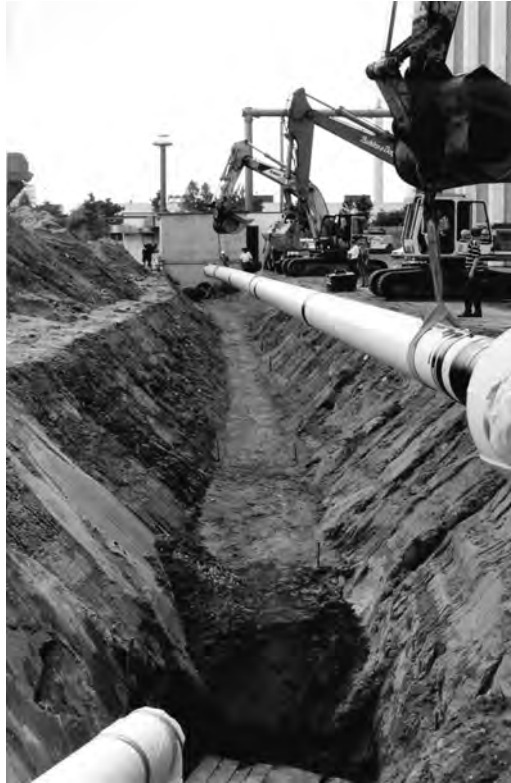
FIGURE 18.20 Trench of 55-m-long section during laying and view into the trench. (Courtesy of Siemens AG, Erlangen, Germany.)
