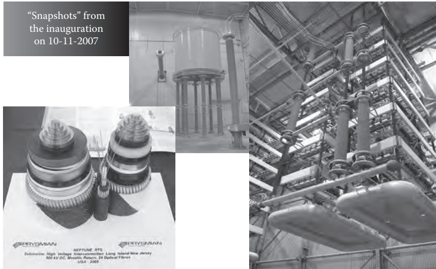
FIGURE 5.6 Neptune HVDC—a view of Station Duffy Avenue inside: the cable, indoor smoothing reactor, and thyristor converter.
