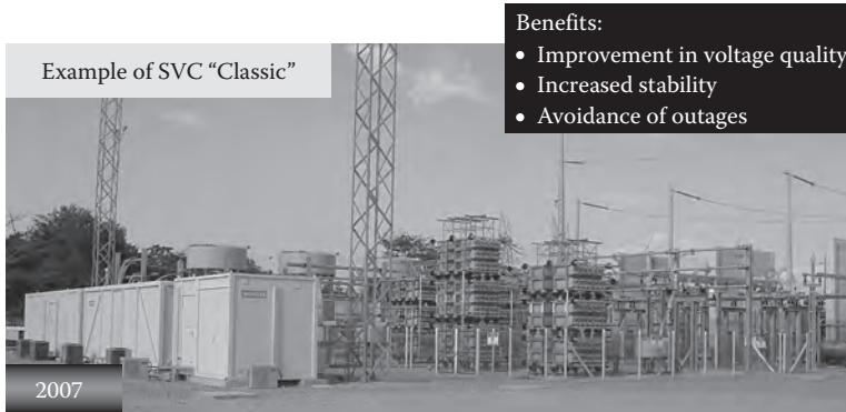
FIGURE 5.24 SVC São Luis, ELETRONORTE, Brazil: TCR, TSC/FC, 230 kV, 150 MVar cap./100 MVar ind.
