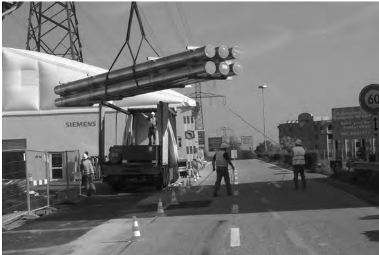
FIGURE 18.26 Delivery of transport unit to the preassembly area. (Courtesy of Siemens AG, Erlangen, Germany.)
