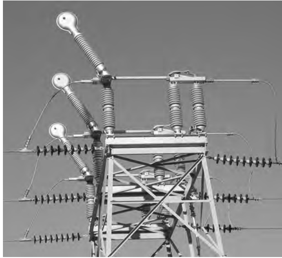
FIGURE 4.27 Load break switch with SF 6 interrupters.
