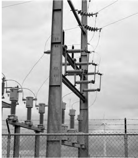
FIGURE 4.31 Incoming line structure mounted power fuses.
