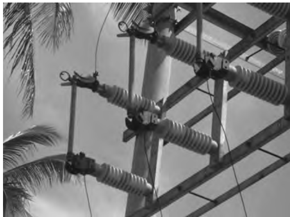
FIGURE 4.32 Vertically mounted power fuses.
