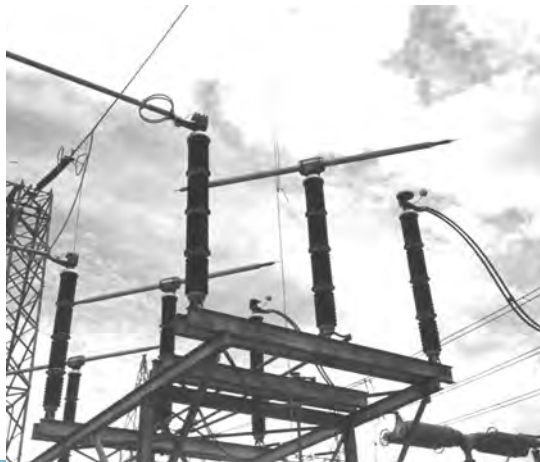
FIGURE 4.21 Double end break disconnect switch in open position.
