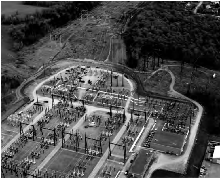
FIGURE 5.36 CSC at NYPA's 345 kV Marcy, New York.
