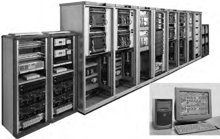
FIGURE 5.39 HVDC “Classic” control hardware—SIMATIC WinCC and SIMATIC TDC (Technology and Drive Control). (Photo courtesy of Siemens AG, Erlangen, Germany.)
