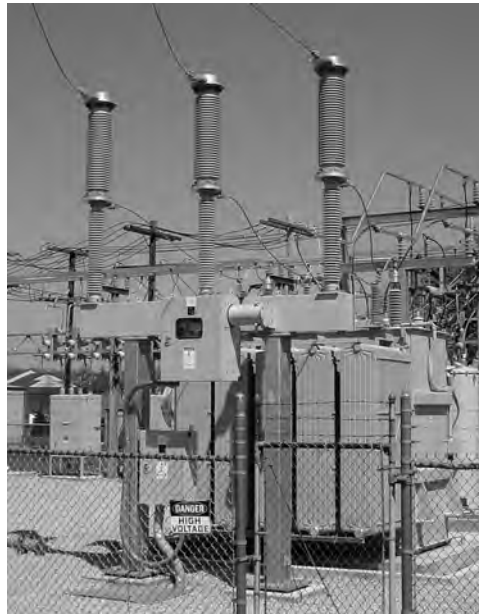
FIGURE 4.34 Vertical interrupter circuit switcher without integral disconnect switch.
