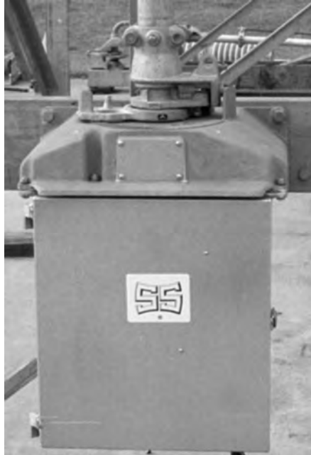
FIGURE 4.6 Motor operator for disconnect switch.
