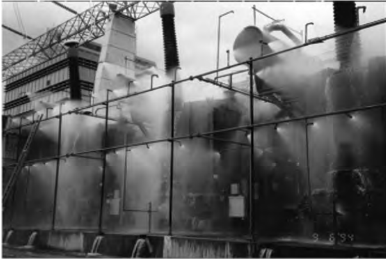
FIGURE 14.5 Transformer deluge system in operation.
