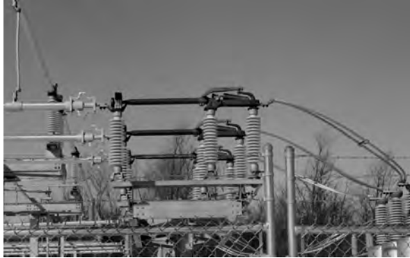
FIGURE 4.8 Horizontally upright mounted disconnect switch.
