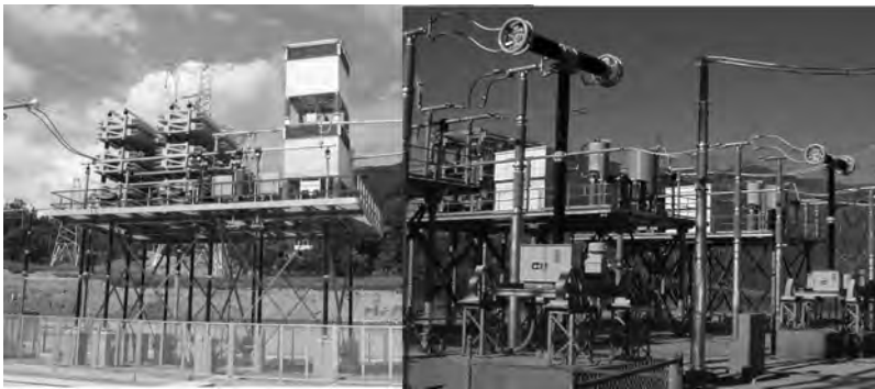
FIGURE 5.28 FSC: fixed series compensation, Fengjie, China, 500kV, 2 \times 610 MVar and TPSCs Vincent, Midway, and El Dorado/USA, seven systems at 500kV.
