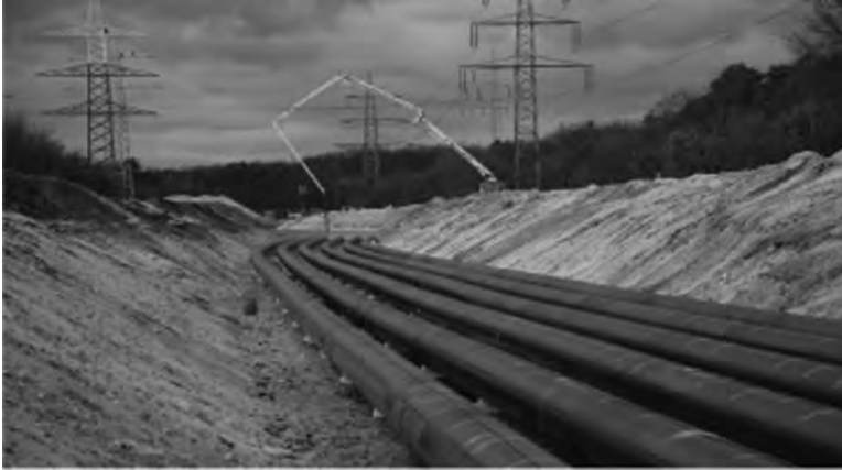
FIGURE 18.28 Two system of 400 kV GIL at the Frankfurt Airport of the Kelsterbach project.
