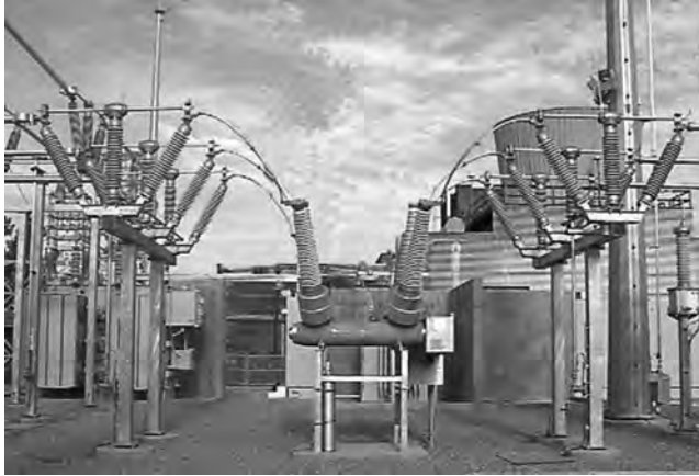
FIGURE 4.22 Double end break “Vee” disconnect switch on single horizontal member, two column structure.
