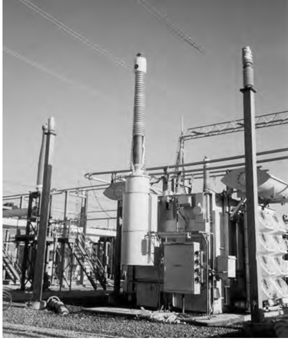
FIGURE 13.3 Porcelain bushing. (Photo courtesy of E. Matsuda, Copyright 1996–2011 Pacific Gas and Electric Company, Oakland, CA. All rights reserved.)
