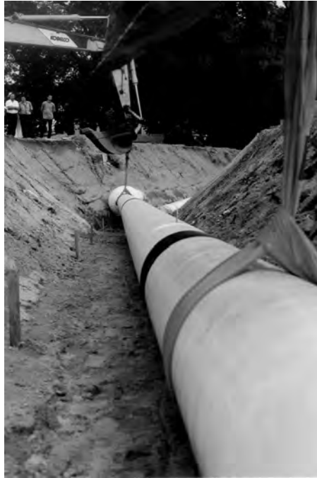
FIGURE 18.5 Laying the GIL into the soil. (Courtesy of Siemens AG, Erlangen, Germany.)
